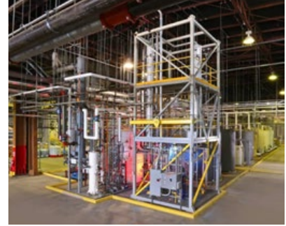
Sandvik will be able to produce tungsten powders in the USA (Courtesy Buffalo Tungsten)
