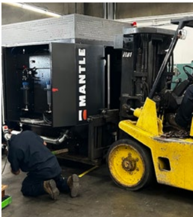
Westec Plastic installing their Mantle metal Additive Manufacturing machine (Courtesy Mantle)
